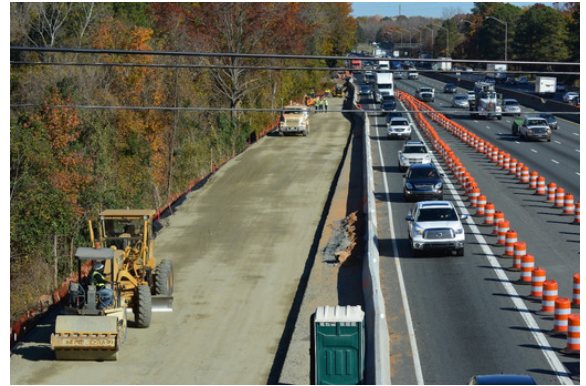
Crews preparing the area and the temporary roadway for the upcoming traffic shifts near uptown Charlotte
